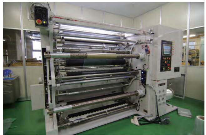
Newly Installed Film Slitter
