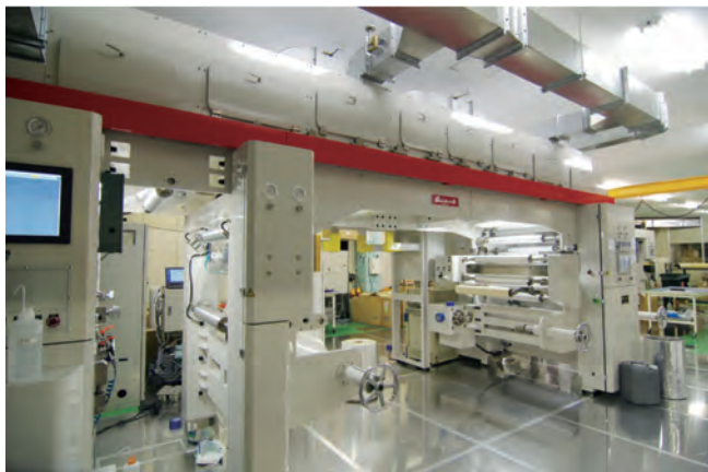
Newly Installed Dry Laminator
